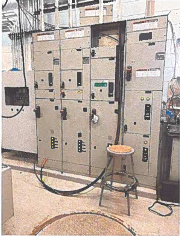
New PLC installation (cabinet to the left)
