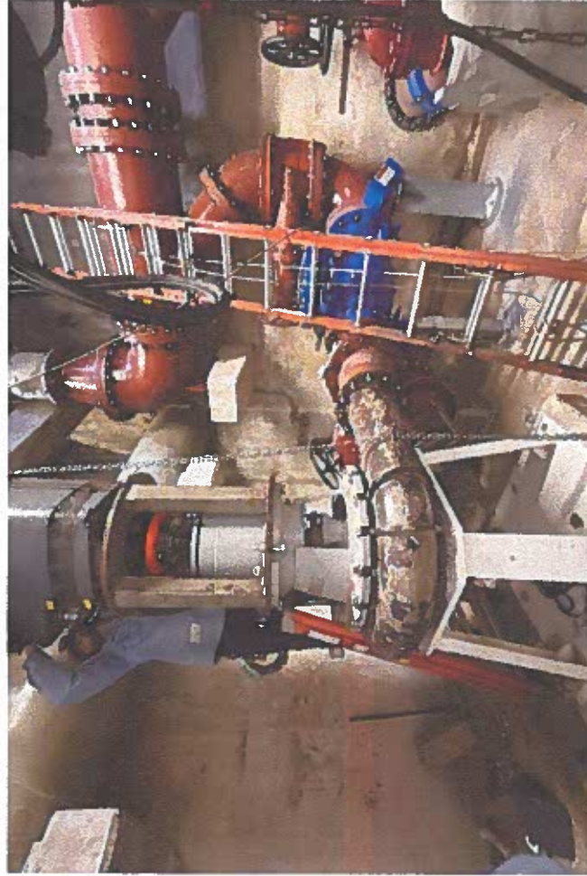
CMCMUA worker mounting salvaged motor upon an existing pump that was re-installed by the Contractor (12-12-23)
