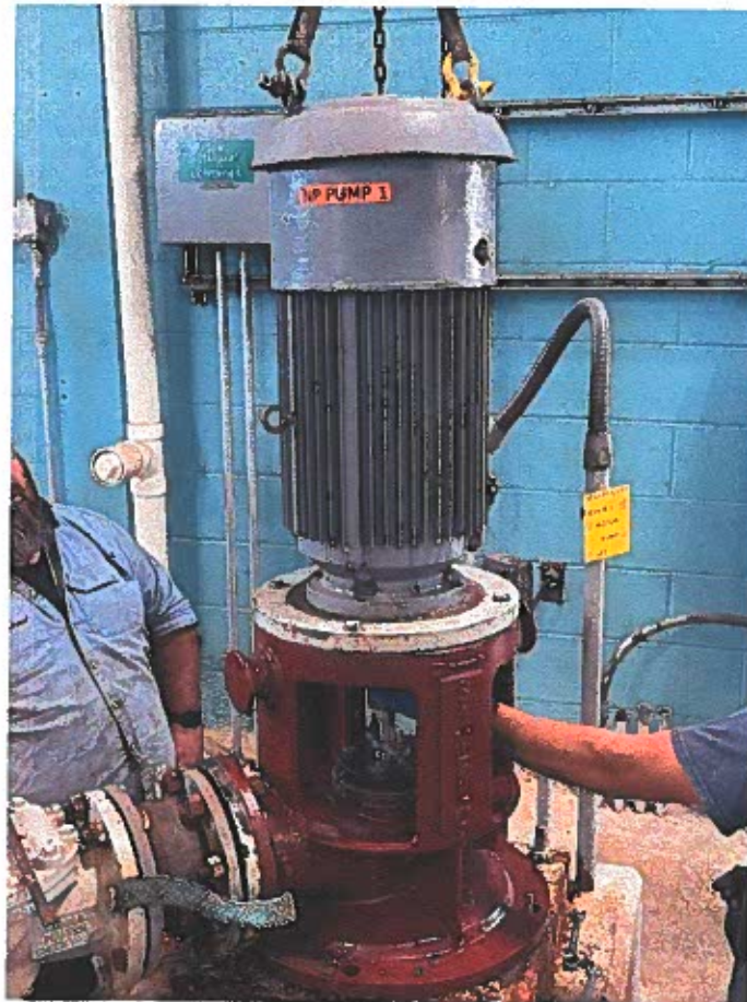
Close up of old pump
