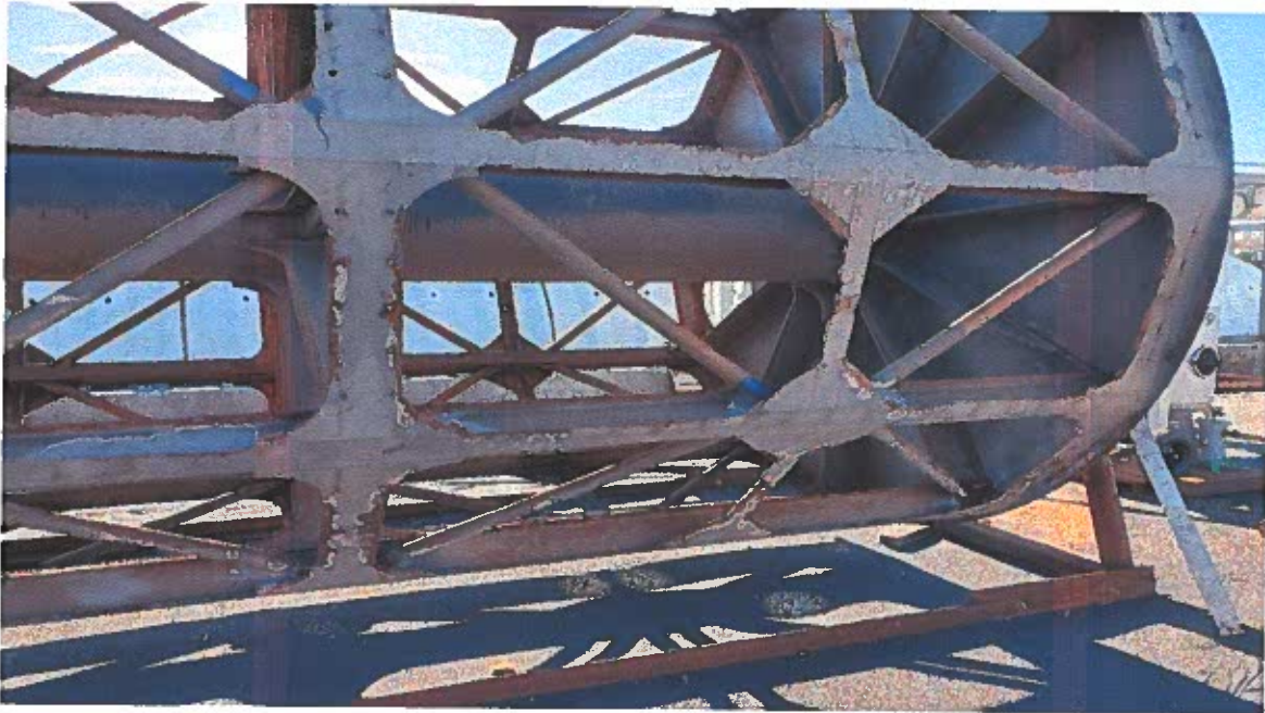
RBR with Repair Areas Noted
