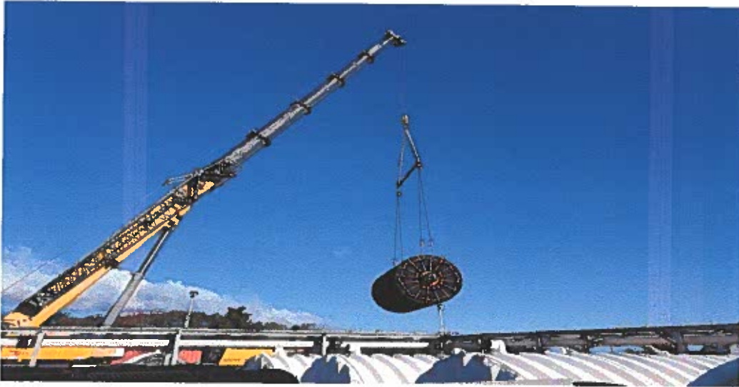
RBC Shaft and Media Removal
