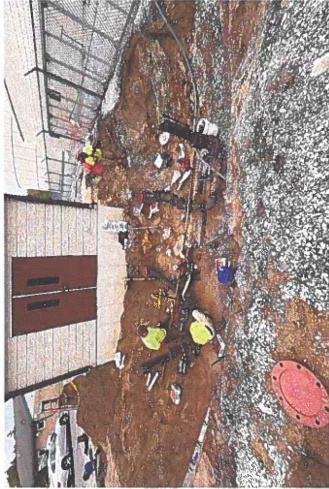
Fire line piping connections (9-18-23)
