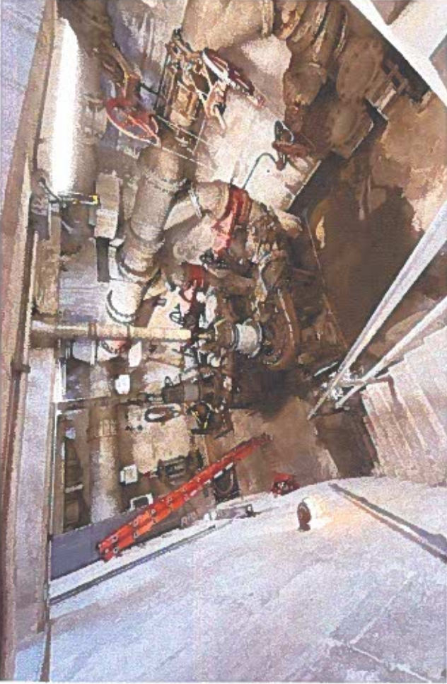
Existing pipe and pump configuration (10-17-23)
