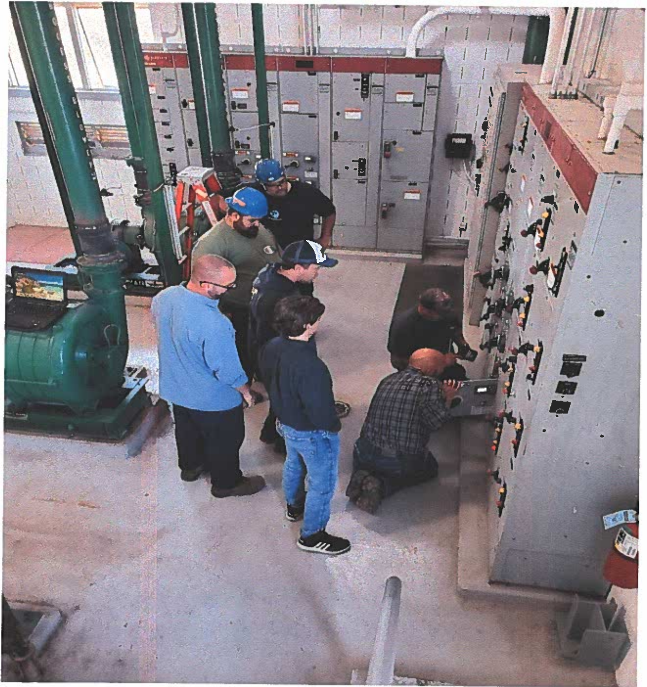
Schneider representatives and CCMUA electricians programming RBC buckets
