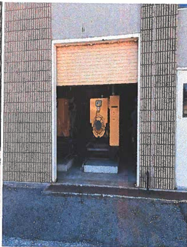
Ocean City generators
