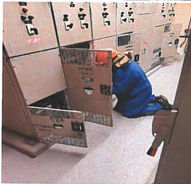
WWL main bus breaker installation
