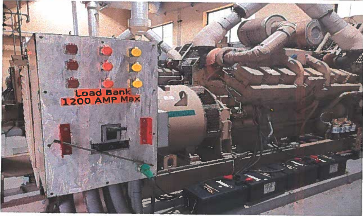
WWL load bank equipment
