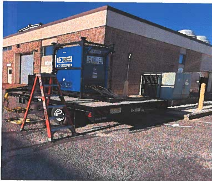
Trailer Mounted Load Banking Setup OC
