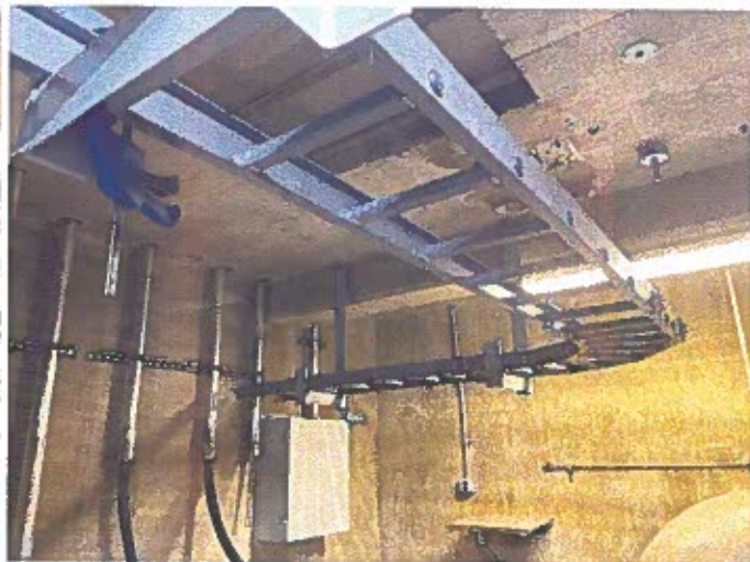
Structure to hold the electrical wires
