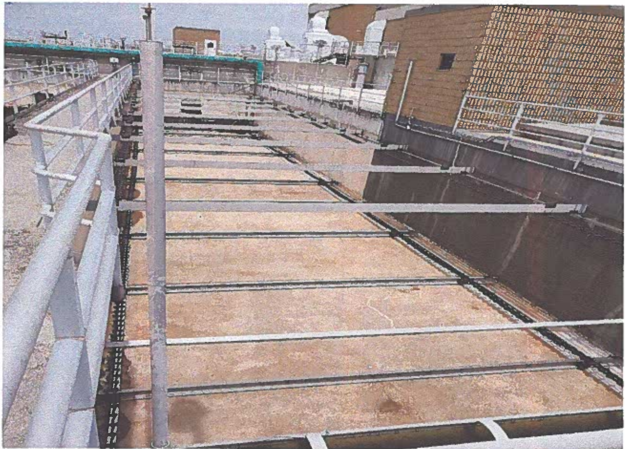
WWL equipment previously installed July 2022
