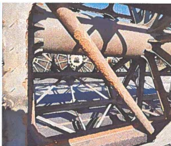
Corrosion of RBR supports
