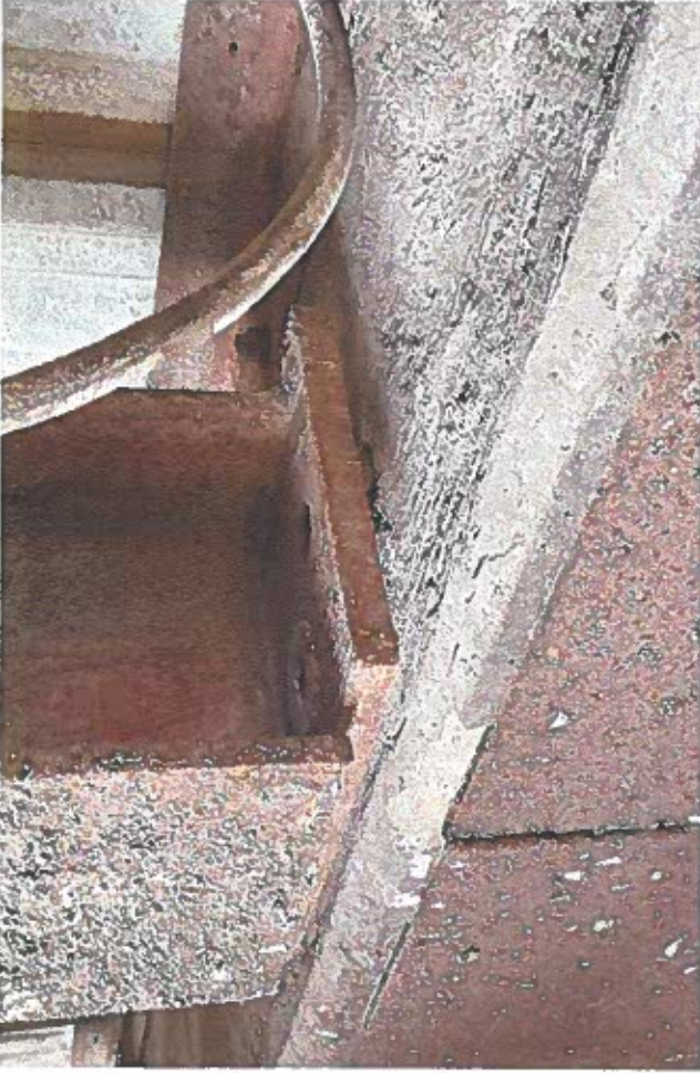
Typical unsupported post base (1-18-23)
