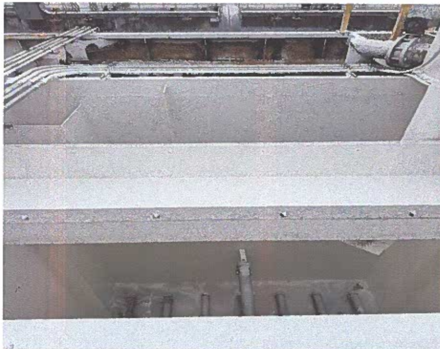
Coating of Filter Cells RWBR
