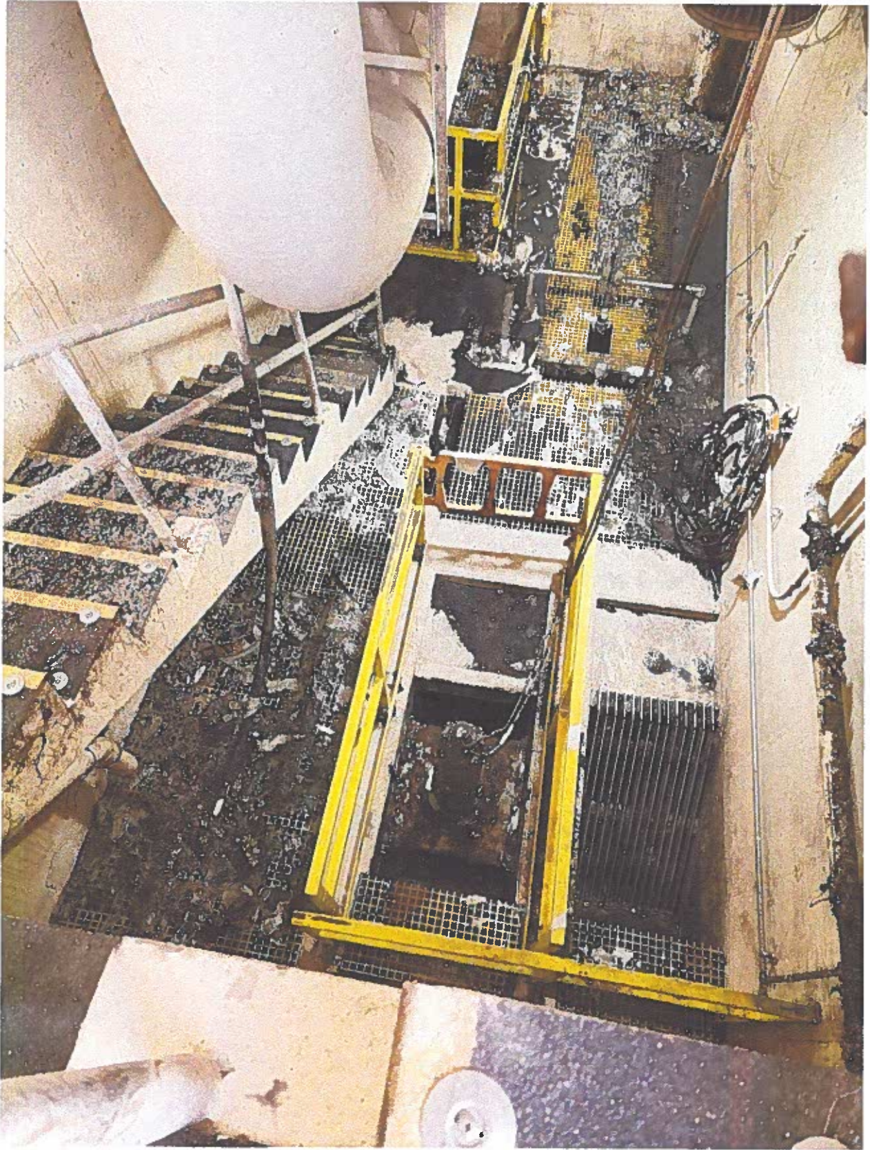
10th Street Pump Station wet well flooding
