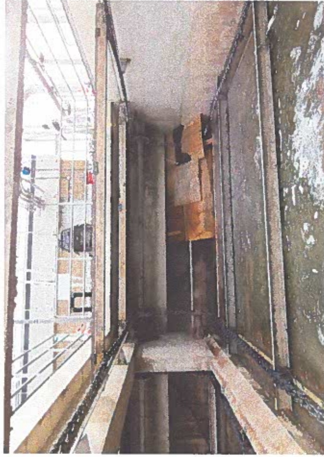
Debris chute to protect clarifier mechanism (1-23-24)
