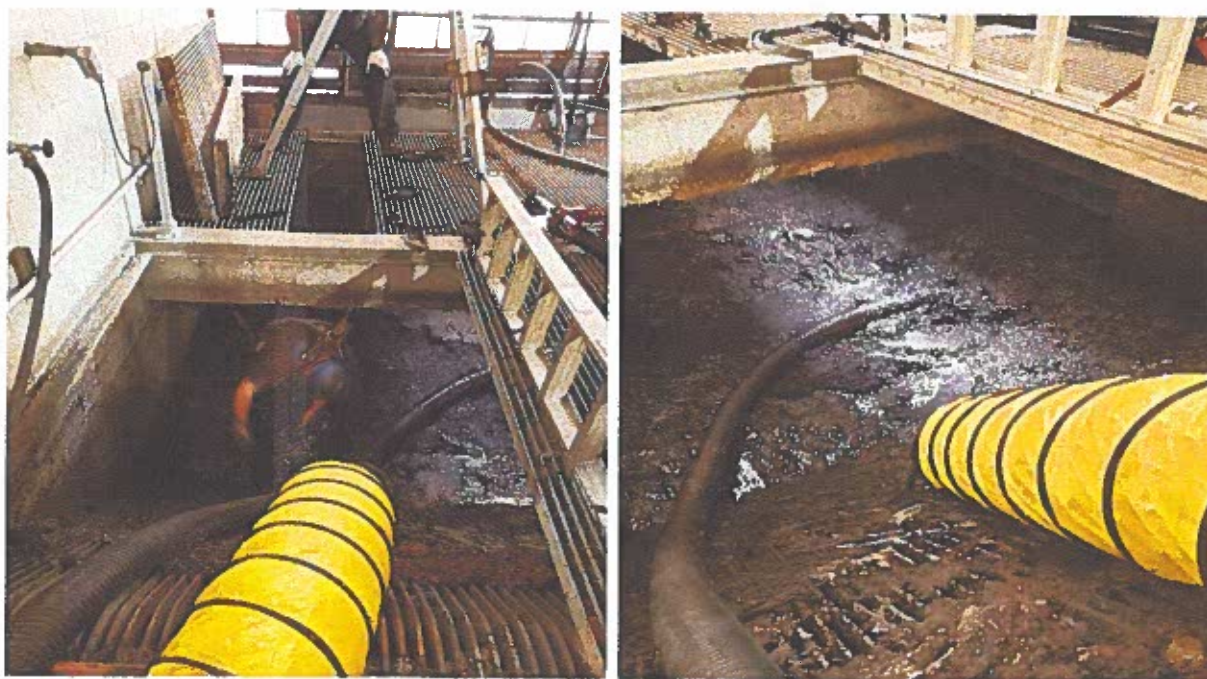
Influent Room Manual Bypass Chamber Vac Operations WW/L
