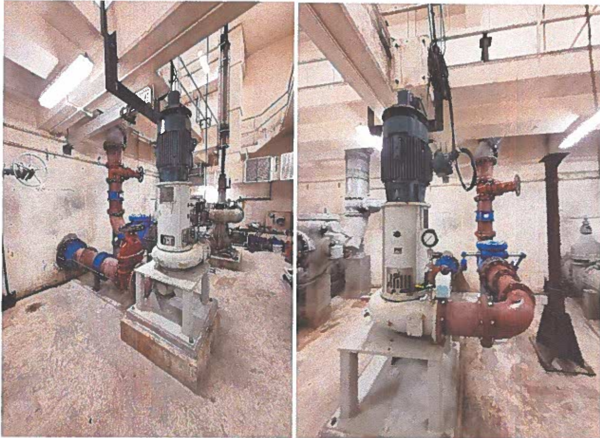
Spicer Ave Pump Station 40 HP Pump Installation (pump motor and red and blue piping are new)
