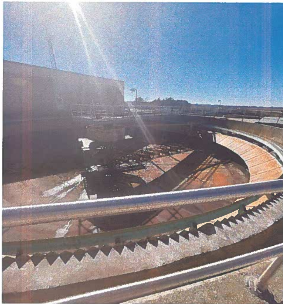
Ocean City Clarifier
