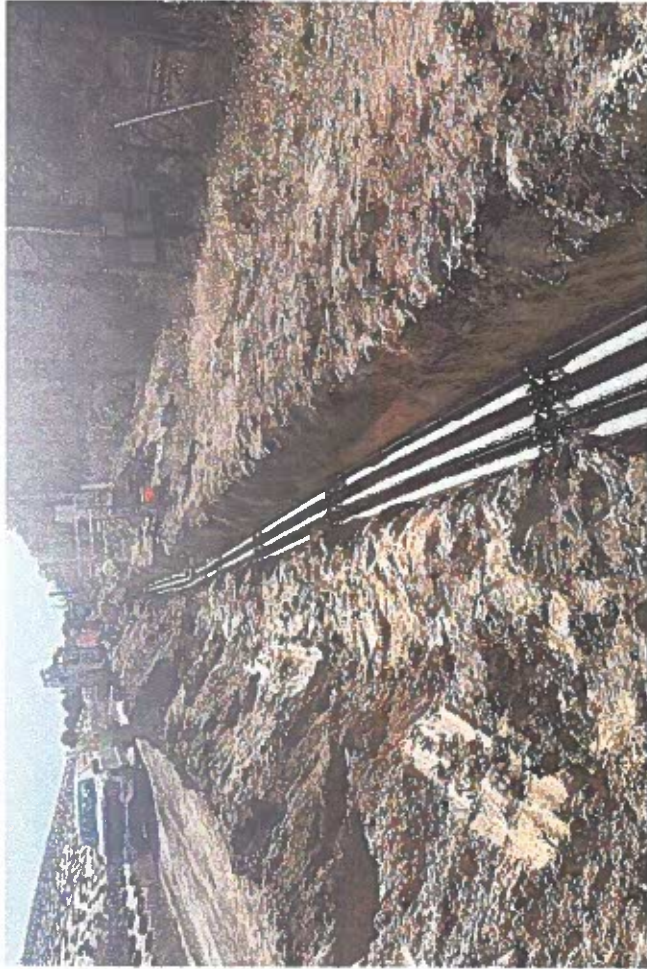
Conduit run from pump Station (2-26-24)
