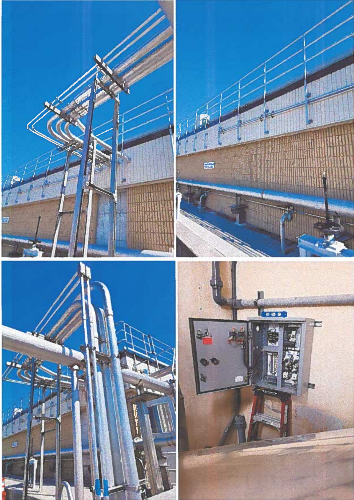
Seven Mile Beach/Middle WTP scum system electrical installation
