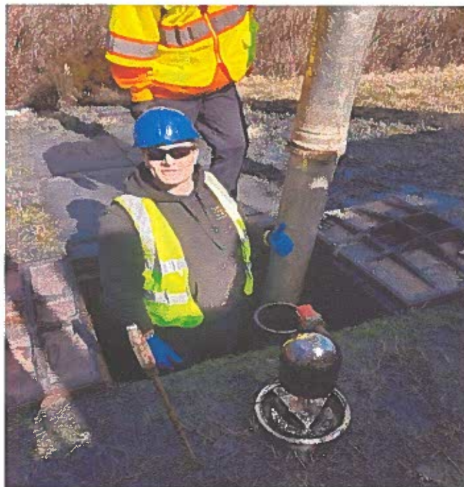
Avalon Blvd air release service
