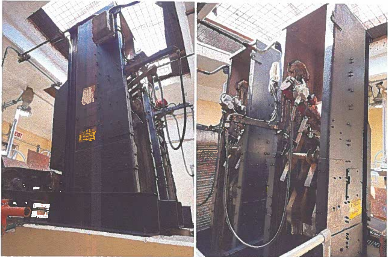
Automatic barscreen coating maintenance
