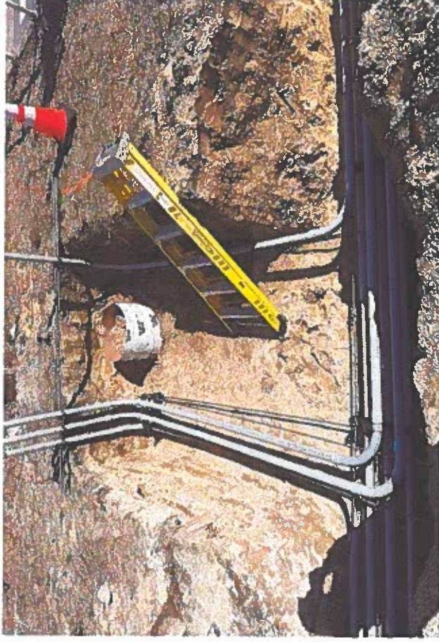
Risers at future backboard location (3-1-24)
