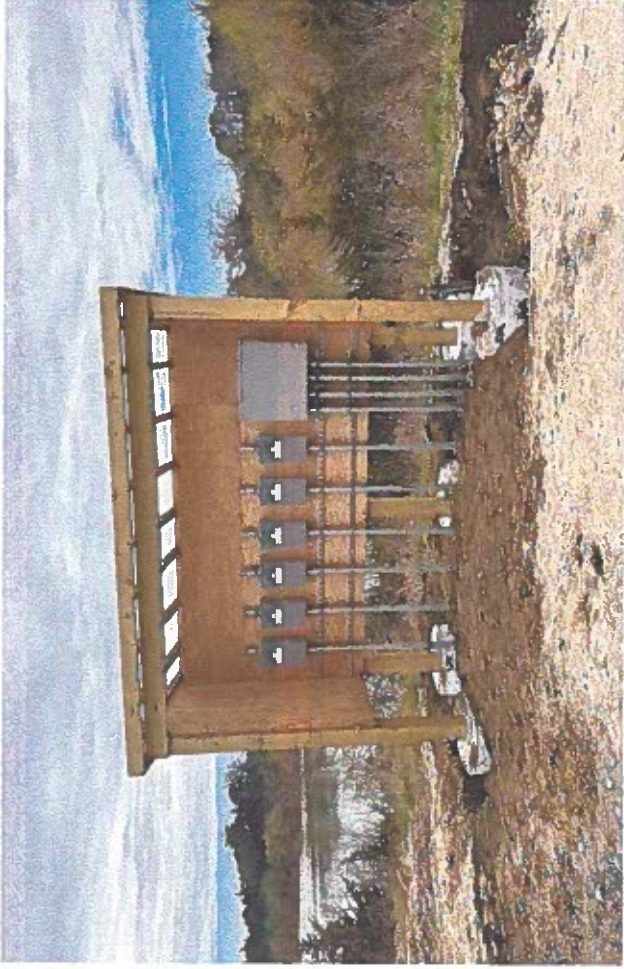
Equipment mounted on backboard (4-10-24)
