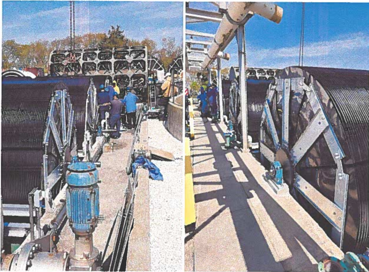
New RBC shafts installed
