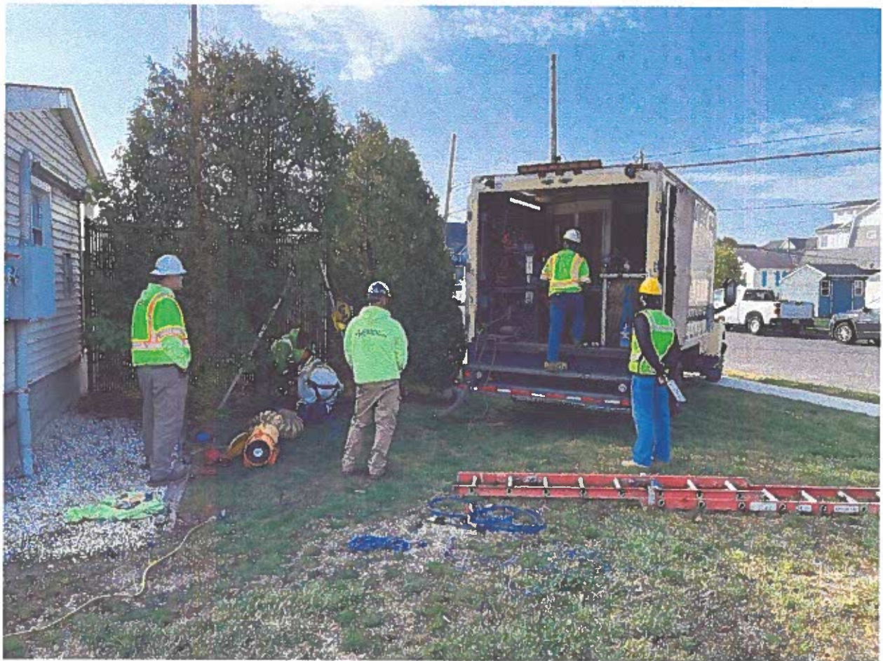
OC 20th St Gravity Line Video Inspections by New Jersey American Water
