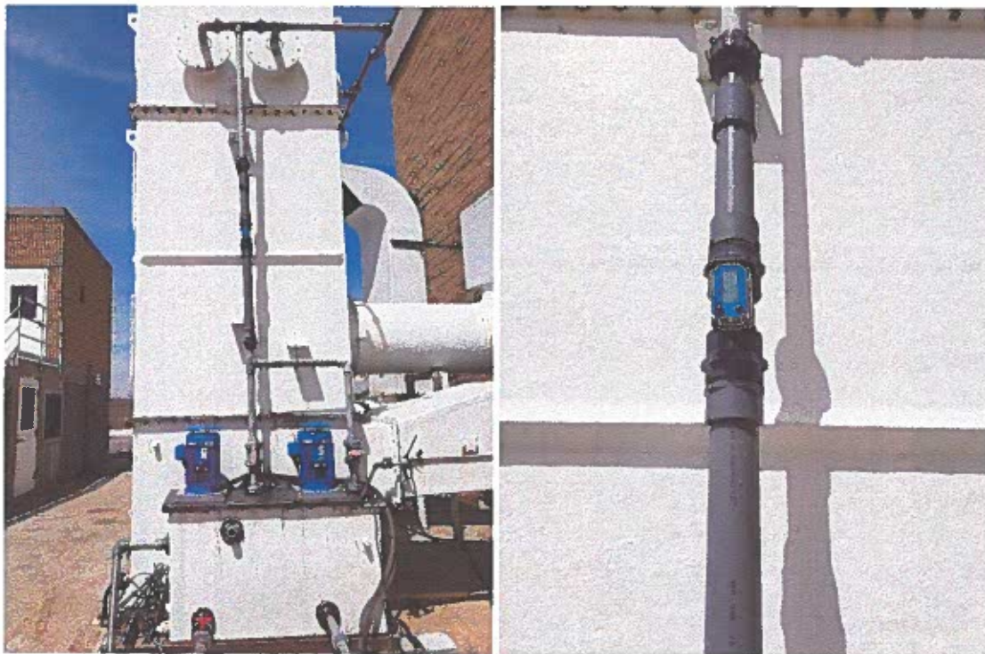
Wildwood/Lower Region Scrubber flow meter installed
