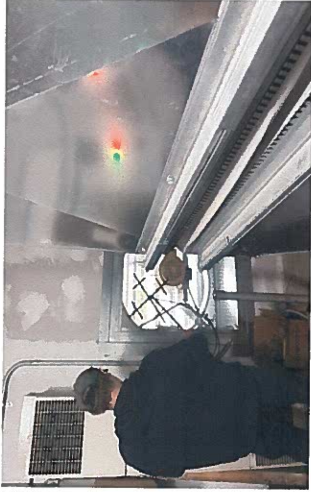
HVAC technician measuring CMCH air flow (5-3-22)
