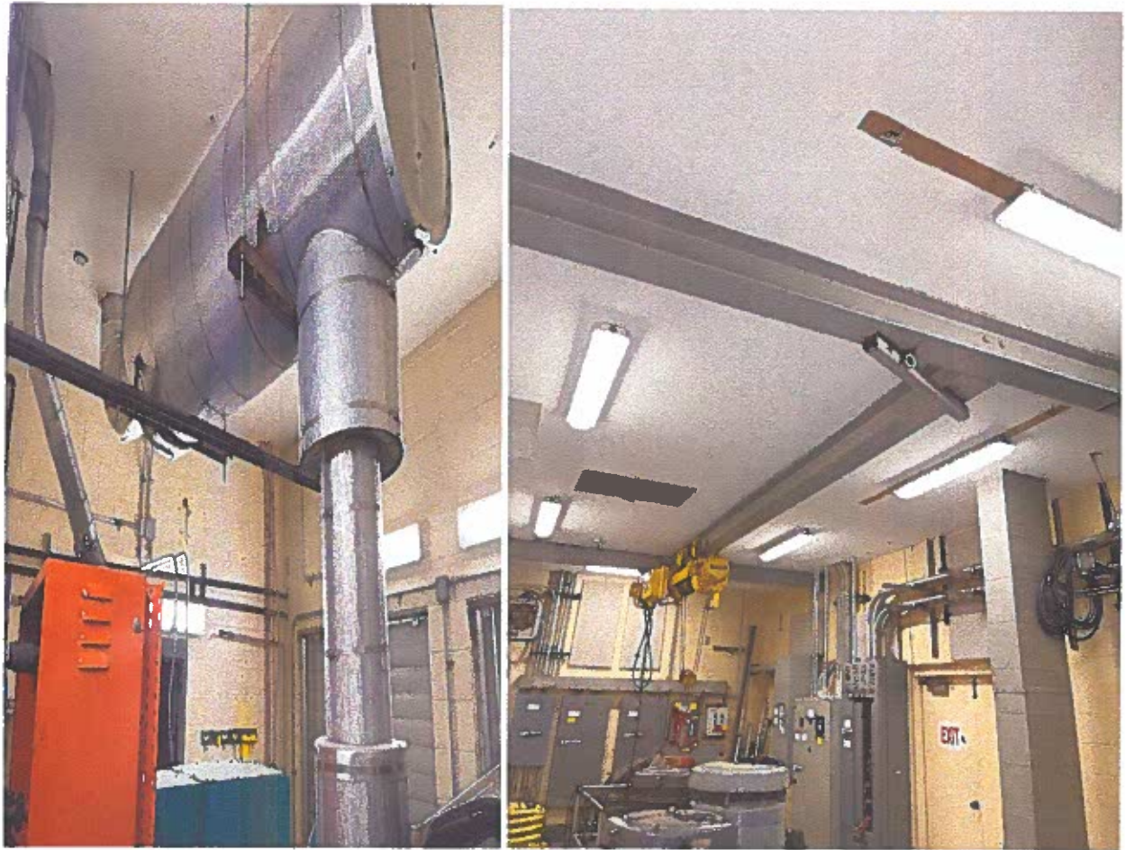
32nd St pump station lighting upgrades
