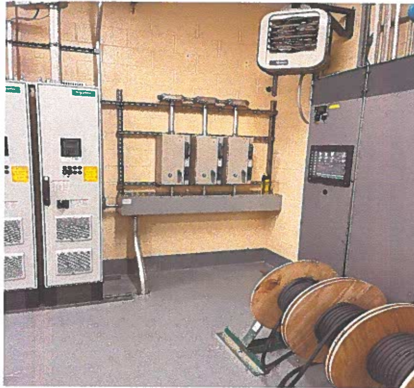
32nd St Cooling Fan Control Panels
