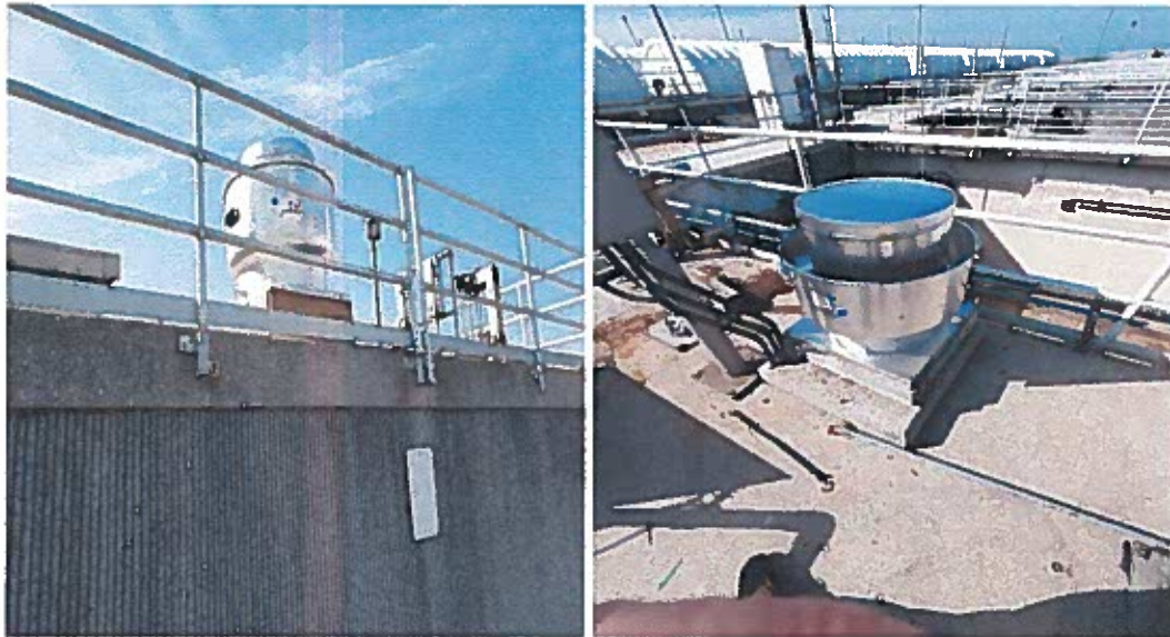
Primary and secondary scum gallery ventilation fans installed
