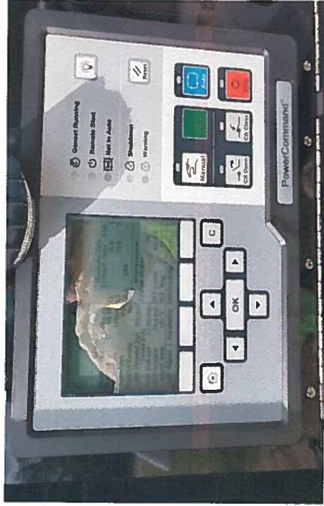
Programming the generator at the Landfill (6/28/22)
