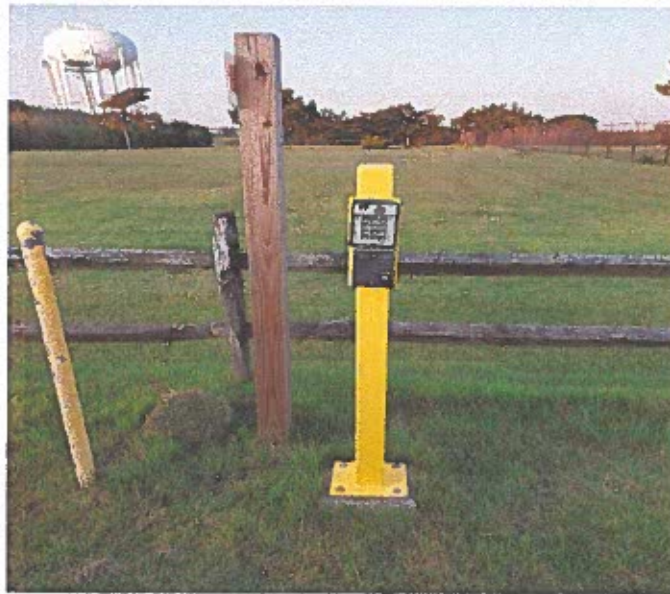
OC gate access keypad
