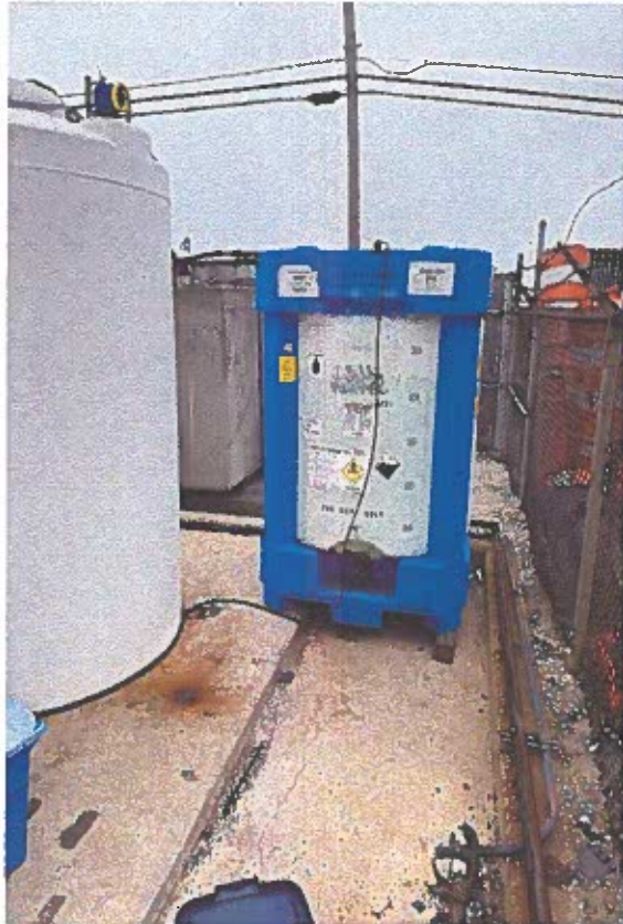
81st Street Chemical Addition
