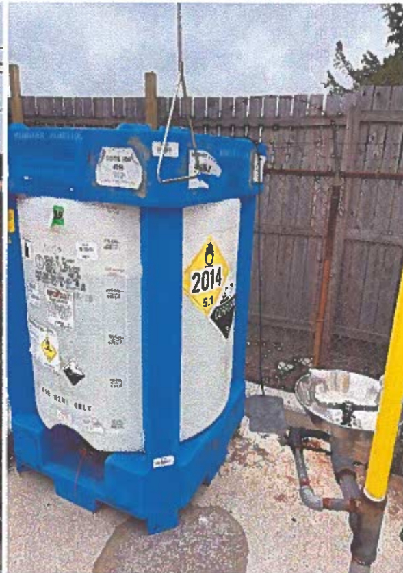
69th Street Chemical Addition
